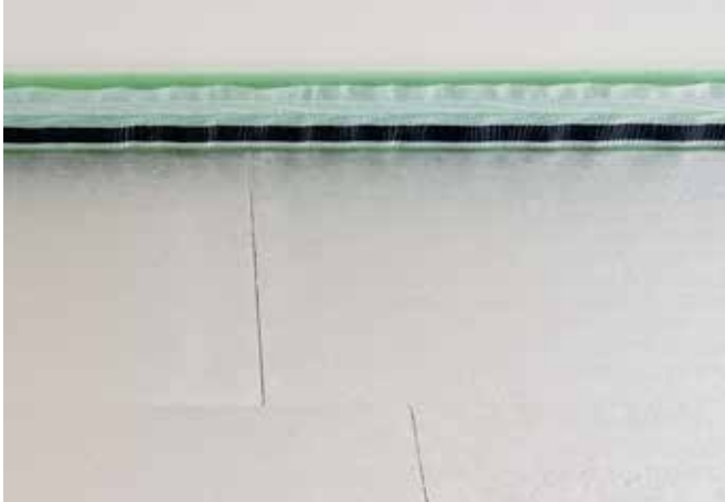
Full-surface laying of the bottom insulation, taking into account the existing supply lines and fixing of the edge insulation strips.
