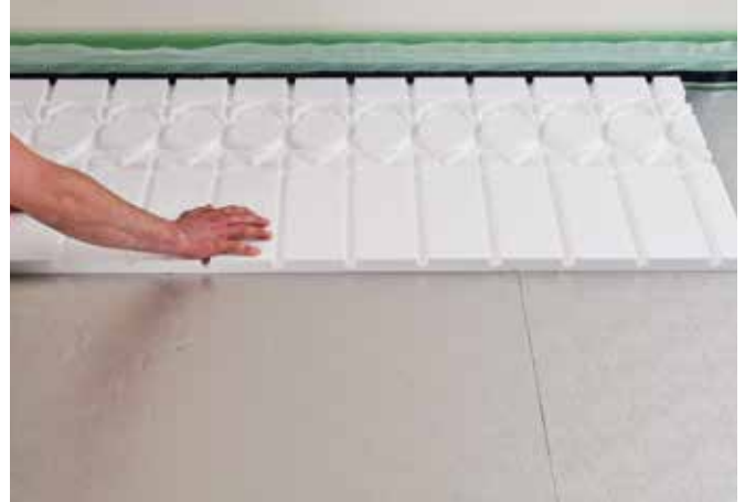
Full-surface laying of the system panels, taking into account the direction of the grooves.
