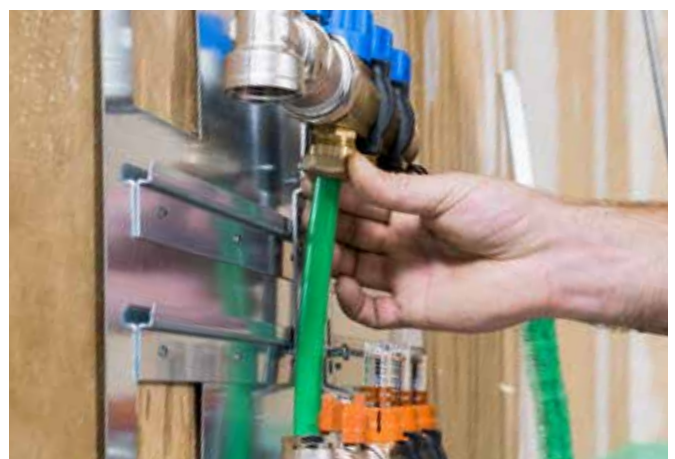
Connecting the underfloor heating pipes to the manifold, filling the system with water and leakage test
