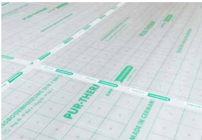
Laying of EMPUR® composite panels. The single-sided film overhang overlaps the connecting panel and prevents the penetration of screed.
