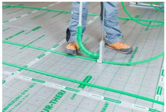
Installation of the KLIMAPEX® heating pipes using the preprinted laying grid with PUR-THERM® staples and the stapler system.
